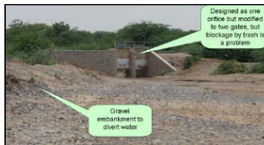
Figure 13. Bagr canal intake
