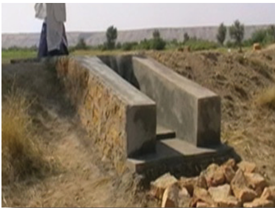
Controlled outflow spillway structure at Motiyo Khan Palari Farm (Sindh) with rocks to dissipate energy at the outlet. Note that a different design is used in EFAP.
