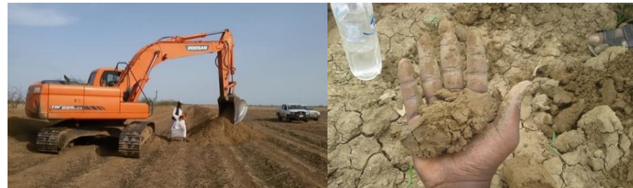
Figure 10: left: construction of mesga canal in GAS, right: soil moisture in GAS one month after irrigating is still high because of more equal water distribution caused by creation of mesga canals.
