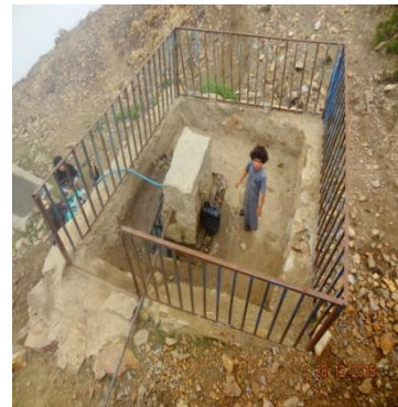
Figure 13 Water Sand Filter
