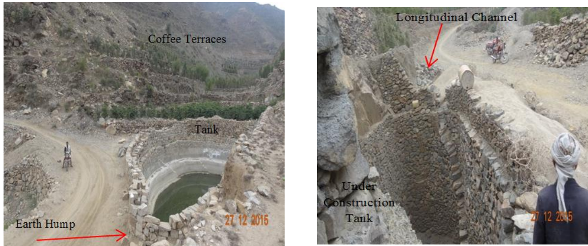
Figure 20 Left: Open water harvesting tank near coffee terraces, Right: Under construction water harvesting tanks
