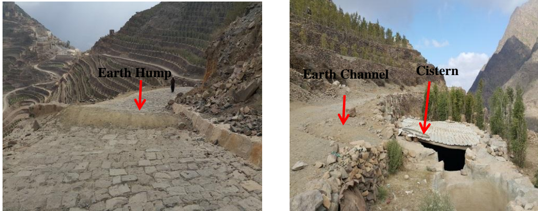
Figure 27 Rainwater diverting earthen humps and earthen channel
