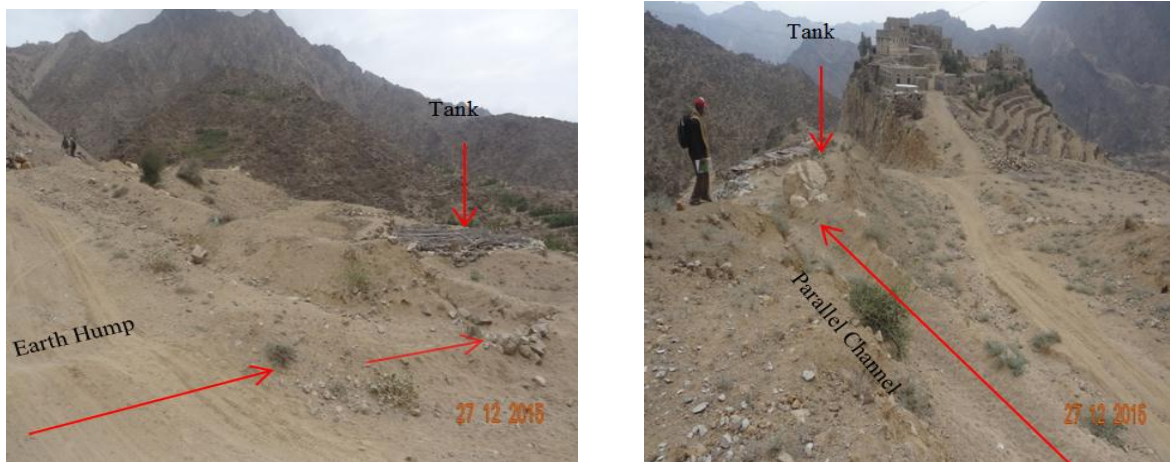
Figure 21 Left: shrubs roofed water harvesting tank the farmer use an earth hump to divert the water from the road surface. Right: old corrugated roofed tank the farmer use parallel side ditch to divert the water from the road.
